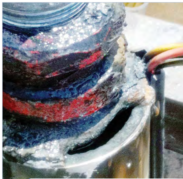
Figure 35. Stray electrical currents formed a hole in this submersible pump. Water was forced through the hole in the bottom of the pump, causing the well screen to collapse and the well system to fail. (Source: Mike Prestigiacomo)
