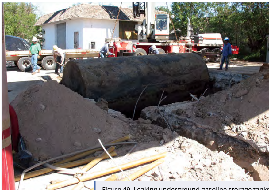
Figure 49. Leaking underground gasoline storage tanks are a common source of groundwater contamination.
